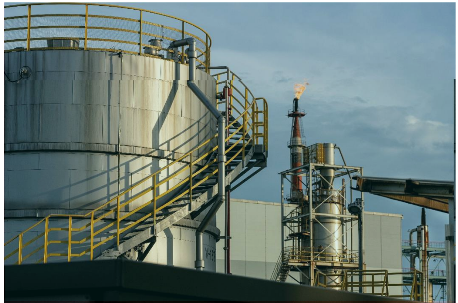
Picture: Tank farm in Lagos Nigeria
